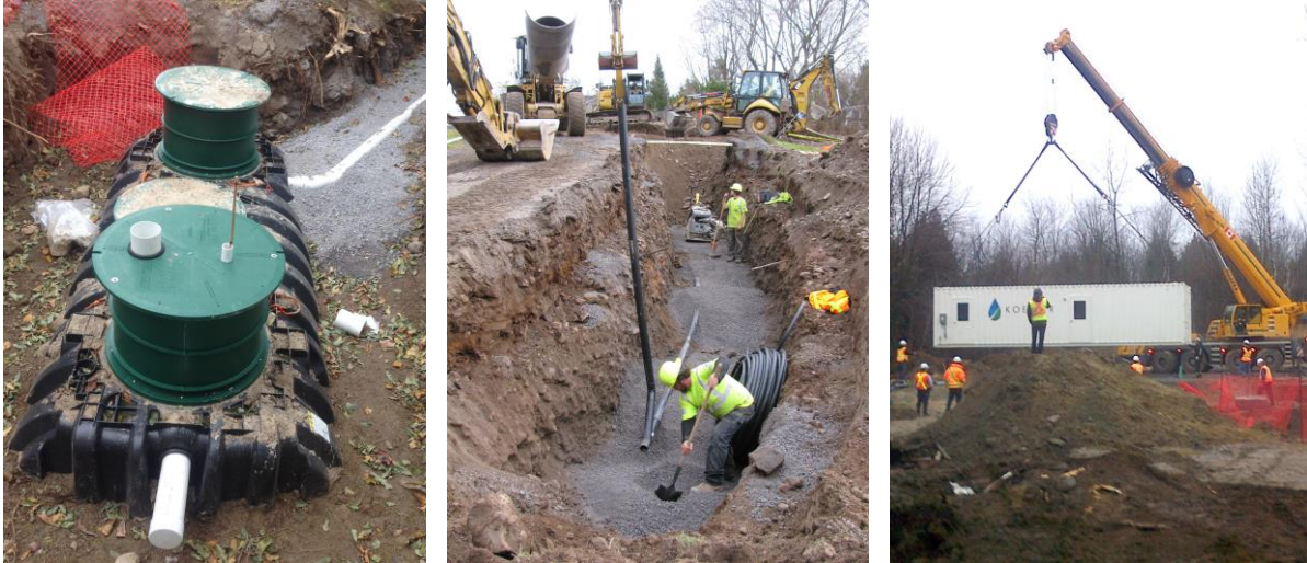
Figures 1, 2 & 3: Installation of an interceptor tank, small diameter gravity sewer and membrane bioreactor in Ontario
