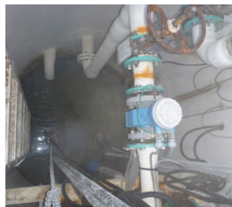
FIGURE 1: SDGS pumping station with minimal solids accumulation after 5 years of operation
