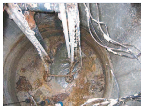
FIGURE 2: Typical raw sewage pumping station with solids and scum accumulation (Environmental Biotech, 2017)
