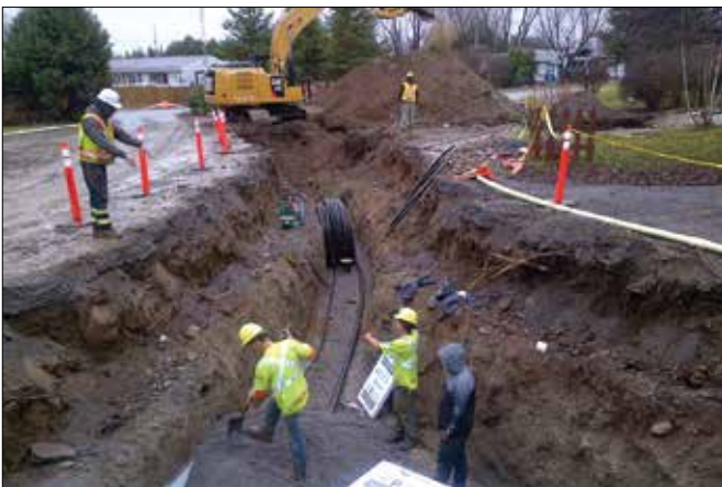
Figure 1 – Installation of a watermain and 75 mm SDGS within a common trench at a mobile home park in Ontario.
