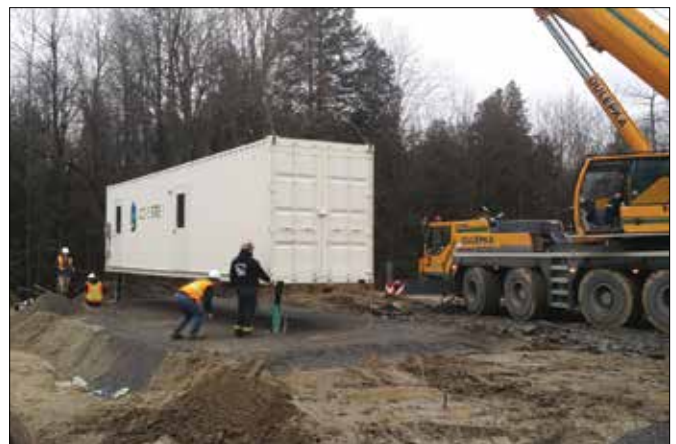
Figure 2 – Installation of the containerized membrane bioreactor at a mobile home park in Ontario.
