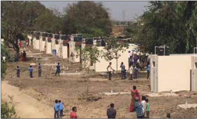
Figure 3 – Constructed toilet facilities and interceptor tanks at a rural village in India.
